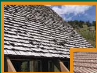
Figure 8: (above) Wood shingle roofs are highly flammable and not recommended. Photo: CSFS
